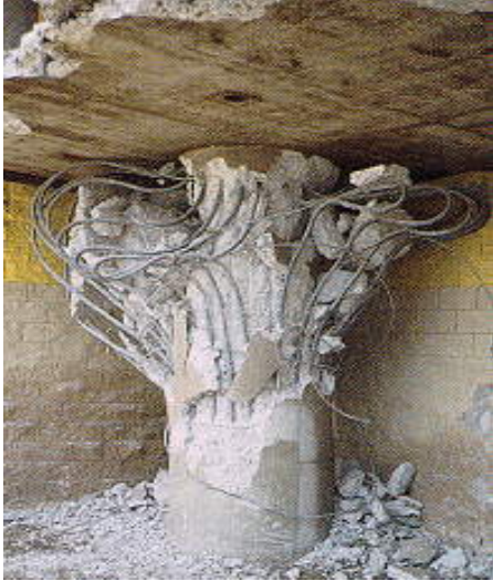
Figure 2: A supporting column of the Santa Monica Freeway collapses.
