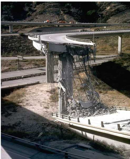
Figure 1: A span of the Antelope Valley Freeway collapses onto the Golden State Freeway below.
