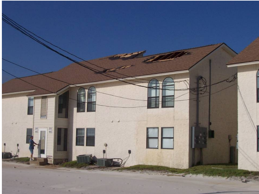
Missing roof sheathing, Gulf Coast of Florida after Hurricane Deniis, 2005.
