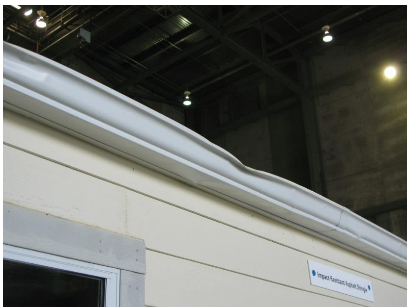
Damage to the specimen house’s aluminum eavestroughs was most pronounced.
