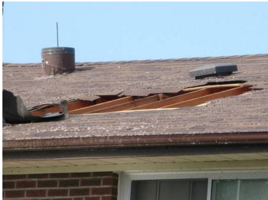
Missing roof sheathing in Vaughan, ON, after an F2 tornado, one of a record 19 that touched down in the province on August 20, 2009.
