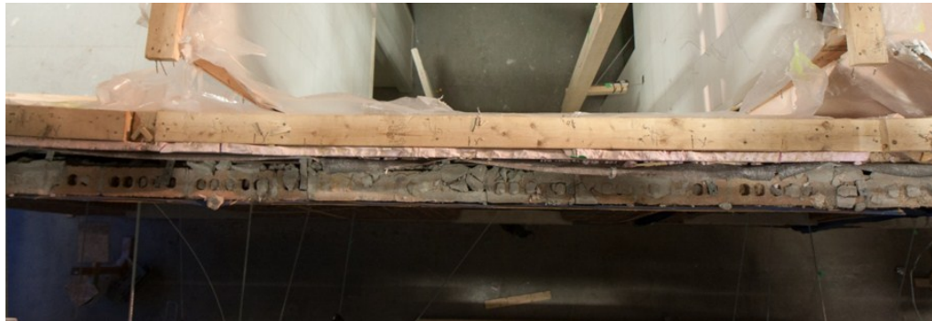
Photographs of the first failure in the brick-clad house, looking down on the wall from above: (upper) at the onset of failure, (lower) and just after failure when the exterior wall was disconnected from the interior walls.
