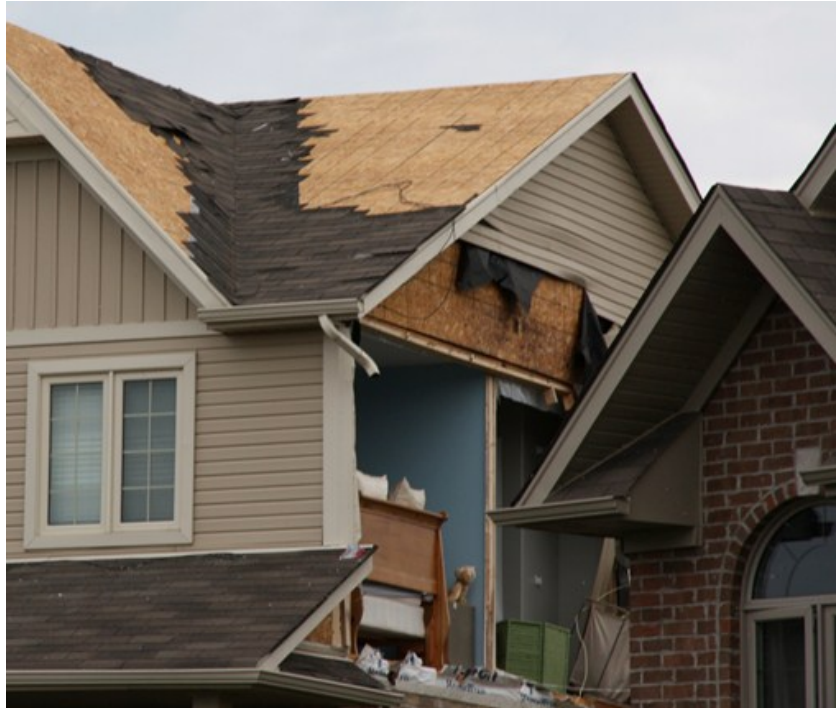
Damage from the Angus Tornado due to improper wall connections
