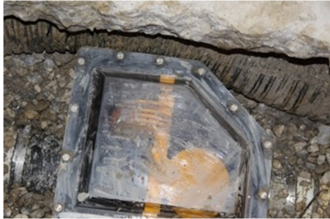
ML-FR4 backwater valve installation in Windsor home.
