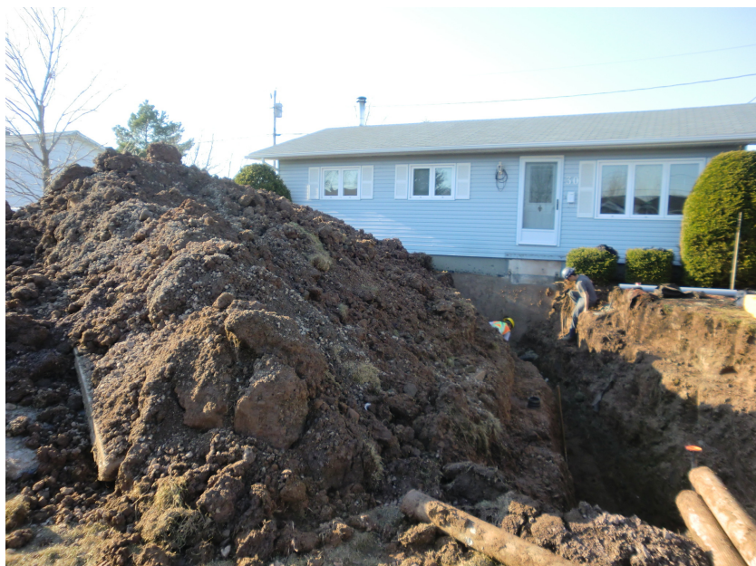
An initial plumbing inspection of the Moncton subject home revealed a major problem with the home's sewer laterals (i.e. the two pipes, storm and sanitary, that connect the home's drainage system to the municipal system).
