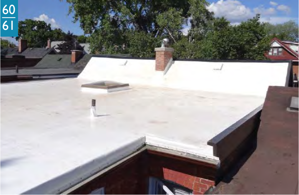
Figure 16: One of the many roofs built under the Eco-Roof Incentive Program in Toronto (Source: City of Toronto)
