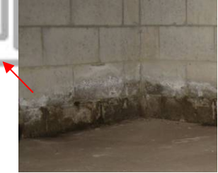
Cracked Basement Wall
