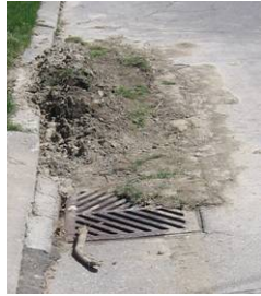
Blocked street catch basin
