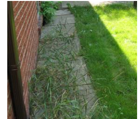
Poor Lot Grading
