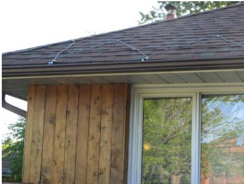
Snow/ice-melt cables were installed on the roof to prevent ice damming.
