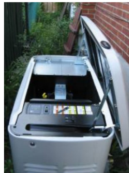
A natural gas-powered generator was installed as an alternative source of power in the event of a blackout.
