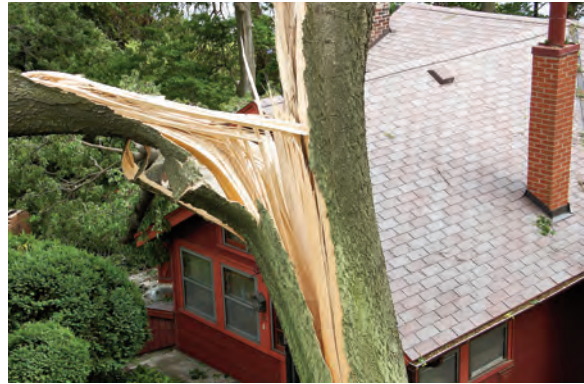
Wind damage in Leamington, Ontario, June 2010.
