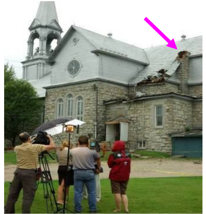
Val-des-Bois Minor damage to chimneys and contents
