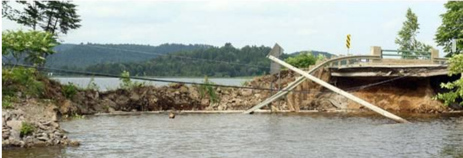
Embankment failure south of Bowman, Quebec. Photograph by: Jean Levac, The Ottawa Citizen.
