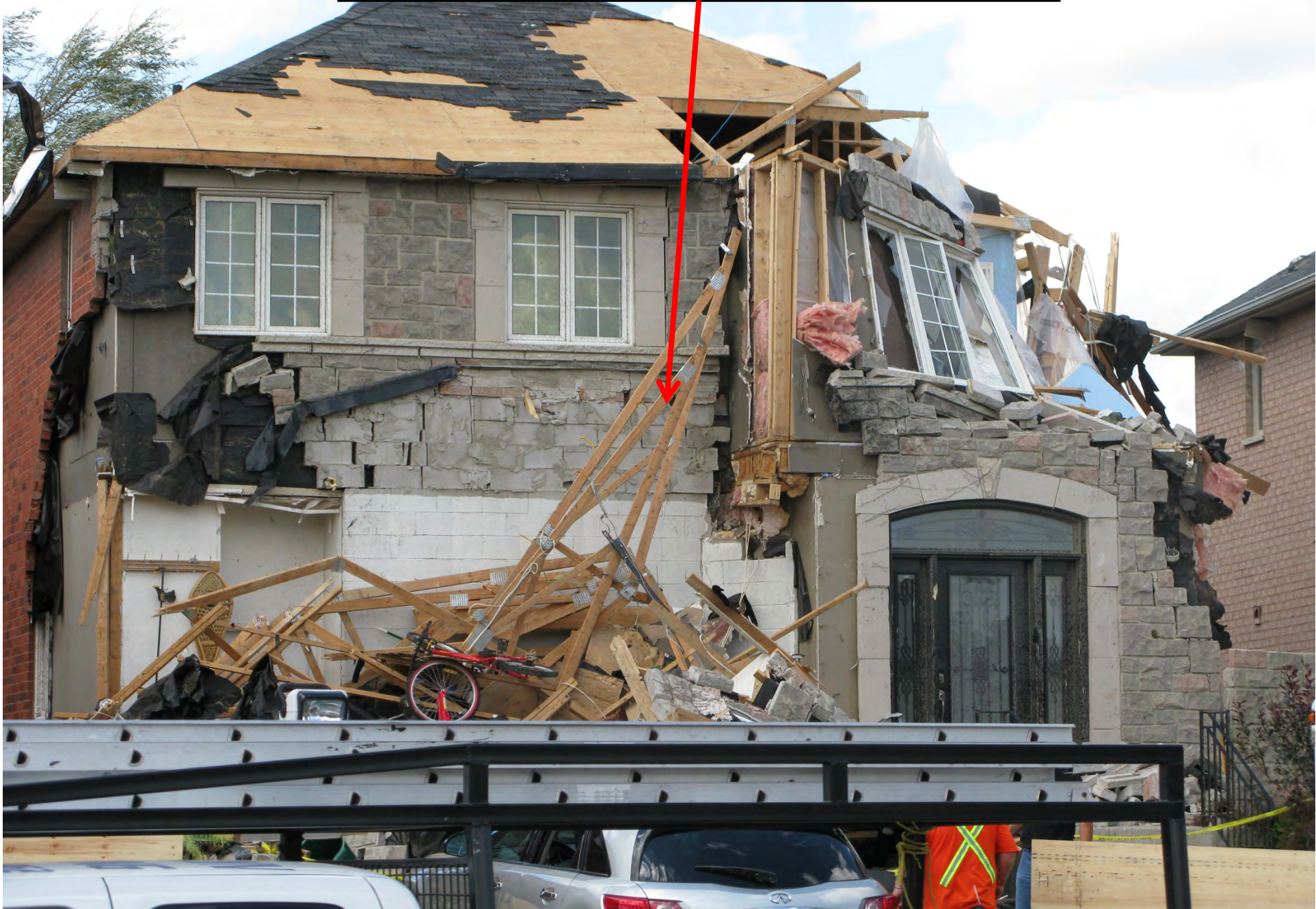
Neighbour's garage roof landed on this house
