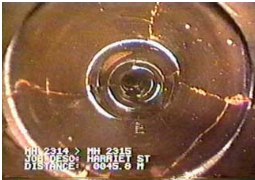
Figure 3. CCTV Scan of a Pipe Section from the City of Winnipeg, MB.
