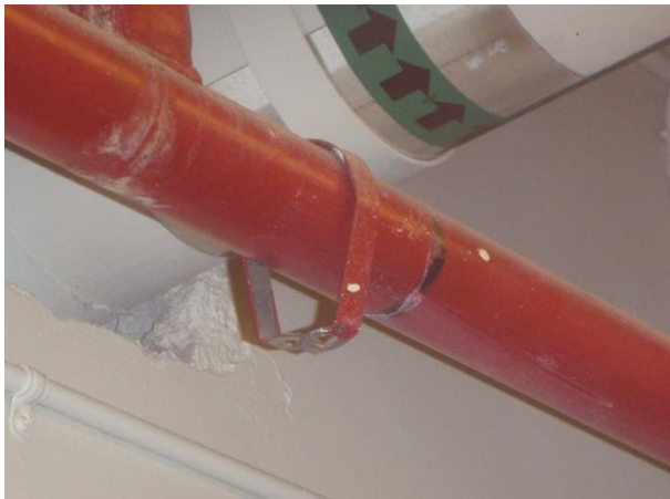
Single solid round rod can bend; Missing supports
