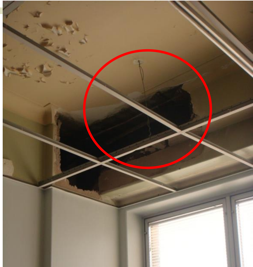
T-bar light framing supported by wires with no lateral bracing
