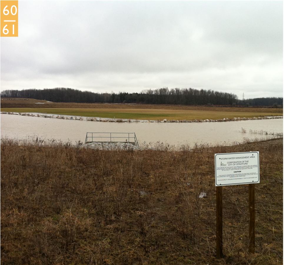
Figure 16 : Stormwater management pond built in Stratford to accommodate surcharging of local systems. (Source: City of Stratford)
