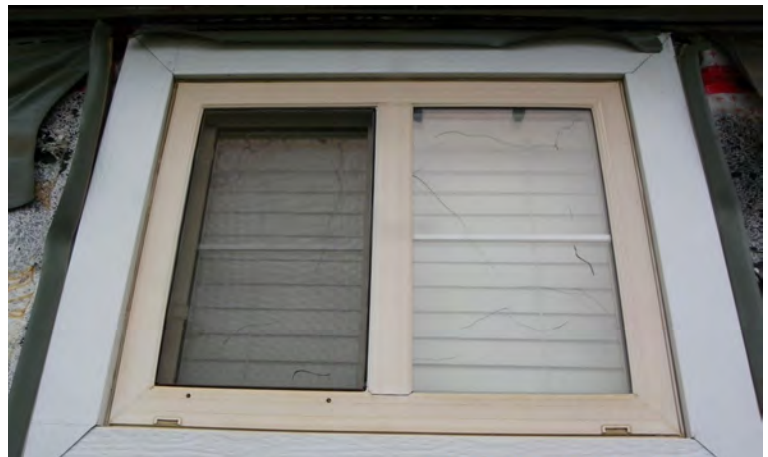
Figure 5-3: Double-pane vinyl mounted windows routinely survived extensive heat exposure
