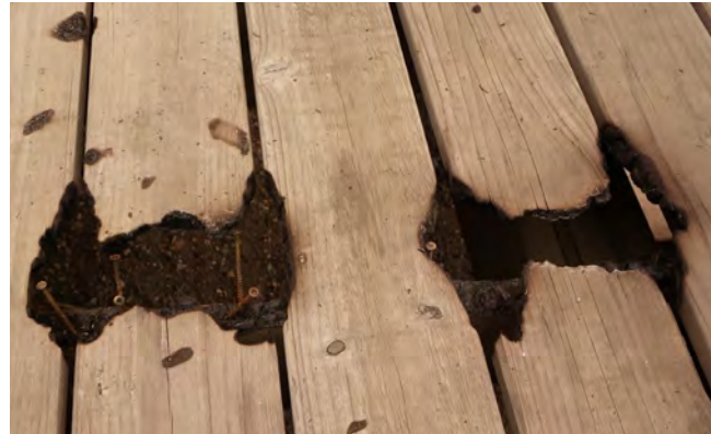
Figure 4-3: Flammable decks and porches were common examples of structural hazard factors
