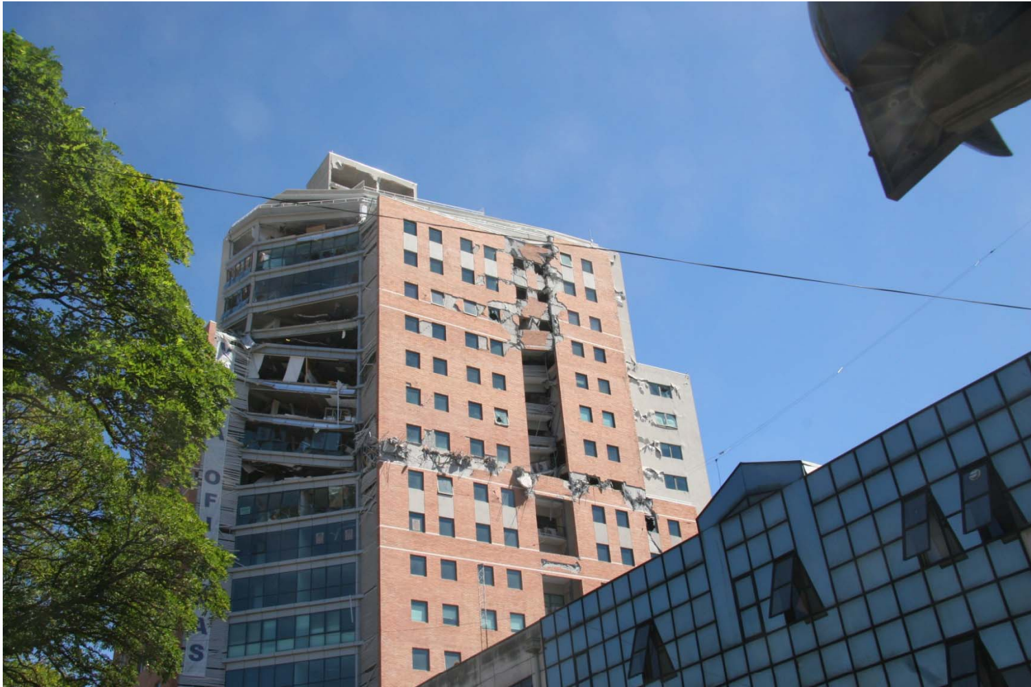
A building in Concepcion: Interstory collapse and will be demolished.
