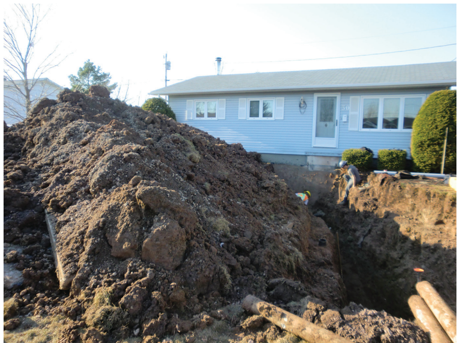
Investigation of sewer backup events sometimes leads to surprising discoveries – as well as extensive remedial work, as shown above.
